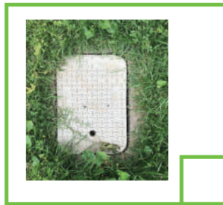
WATER METER BOX
