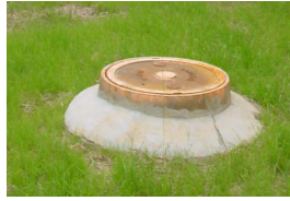
RAISED MANHOLE COVER
