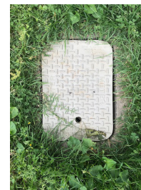
WATER METER BOX
